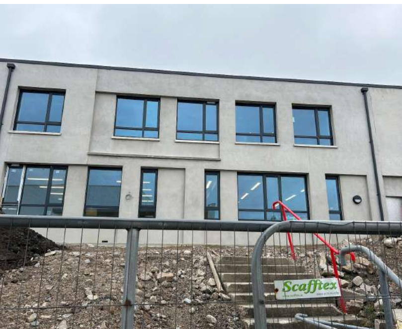
The finishing touches to the first phase of the new buildings are in completion with windows, plastering, lighting and soffit in place now.
