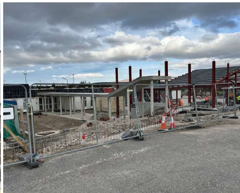
The new front entrance to the RCS and new classrooms to the right of it are now gathering pace in their development.
