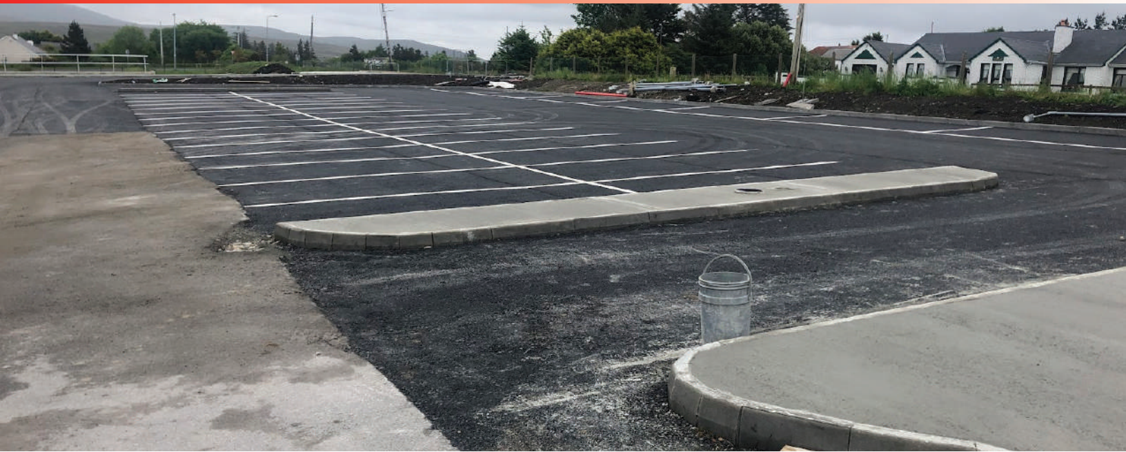
The new car-park is taking shape on the grounds of the RCS.
