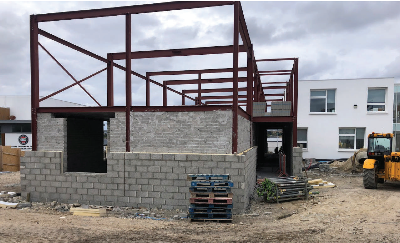
The new buildings project has gathered pace in April and May as new classrooms are on their way!
