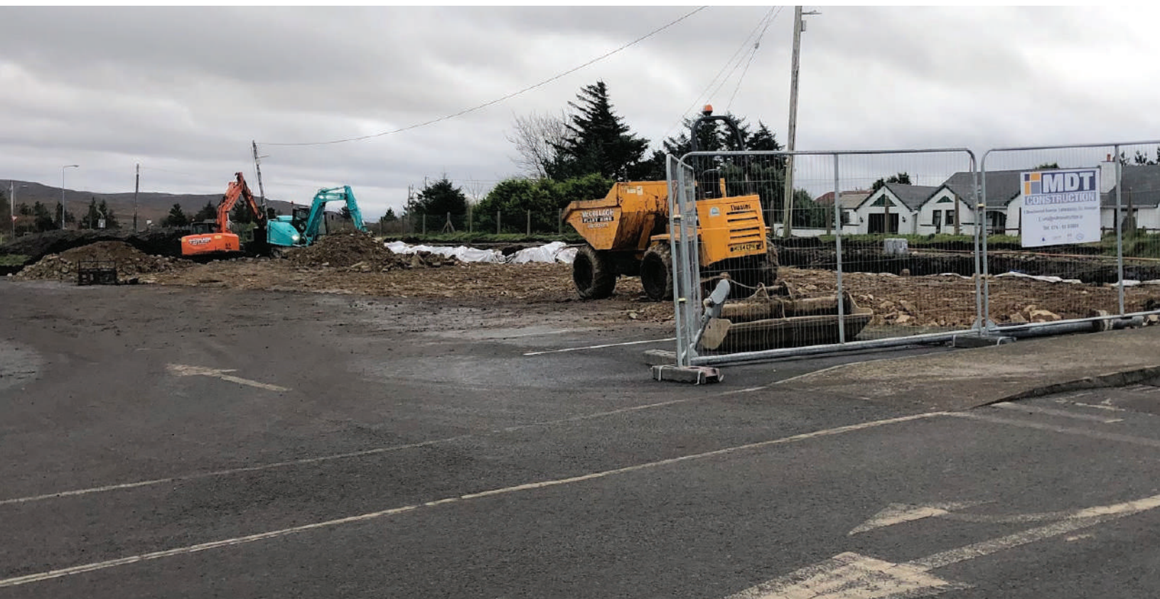
Works have commenced in recent weeks on the new buildings development within the RCS.
