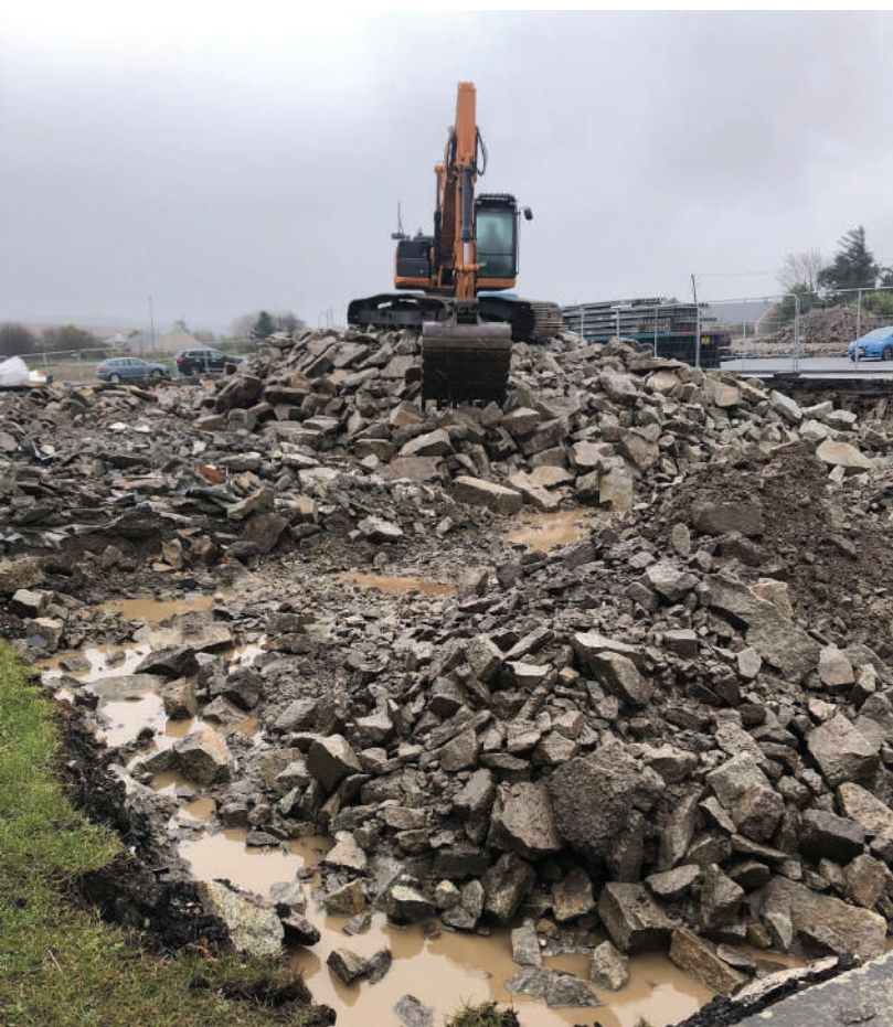
Since January, the school has said 'goodbye' to some old classrooms as work commences on the new buildings project.
