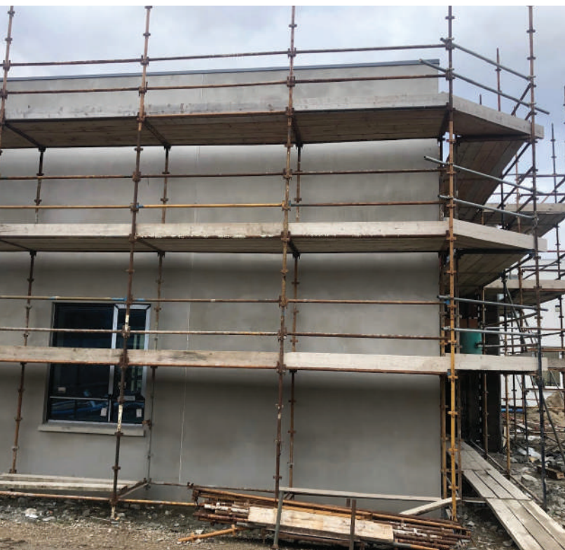
The new buildings near the gym have made good progress in recent months. Windows, plastering and wiring are all in process.
