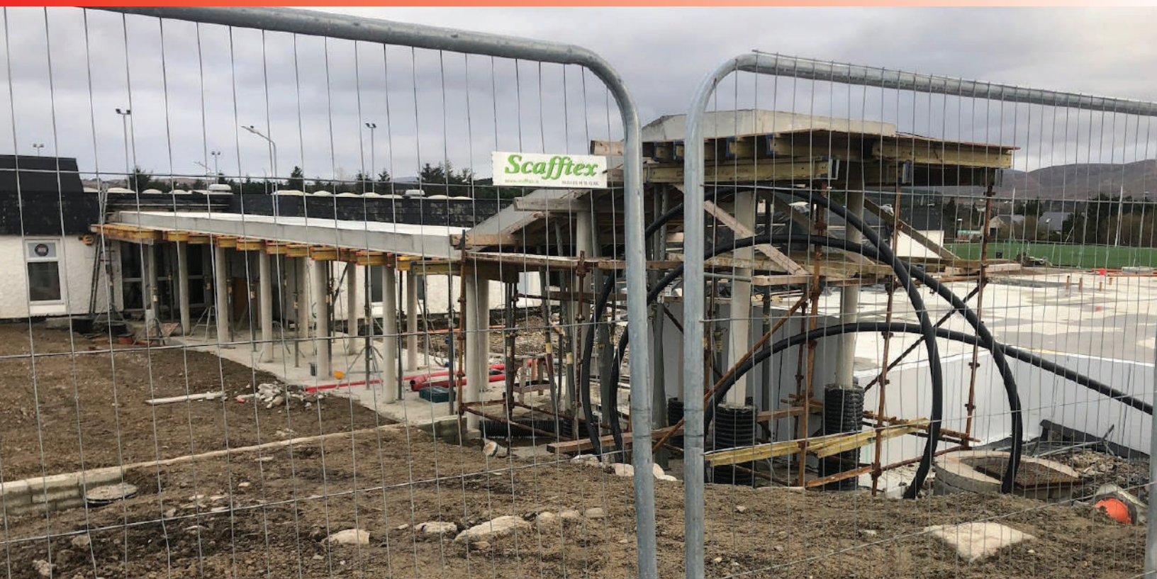
The new front entrance to the RCS is beginning to take shape.
