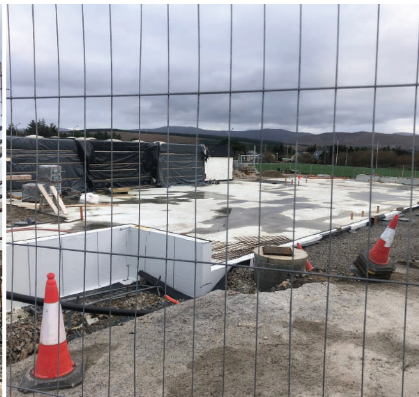
The foundations of many new classrooms to the right of the entrance are now in place and blockwork will proceed shortly on this phase.
